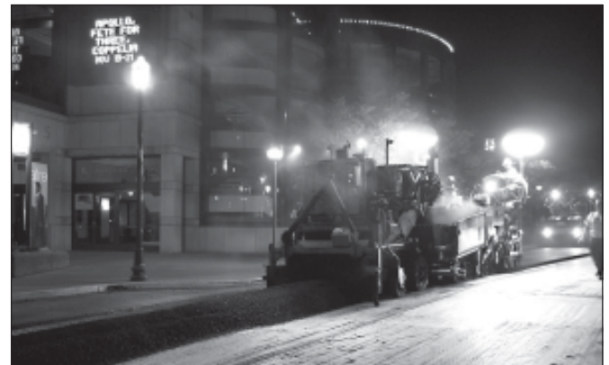
The Civic Drive rehabilitation project got a boost from Federal Economic Stimulus money.
